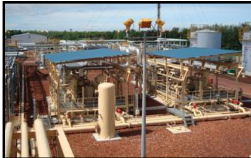
Sangu Gas Compressor Project (Cairn Energy) (Commissioned in July 2009)
